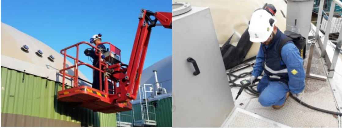
Photo A15.2: Leak detection measurements; confirmation of a biogas leak by FID
